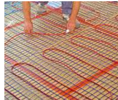
Heating cables connection.
